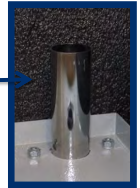
Temperature probe installed. Temperature control activated at 30°F
